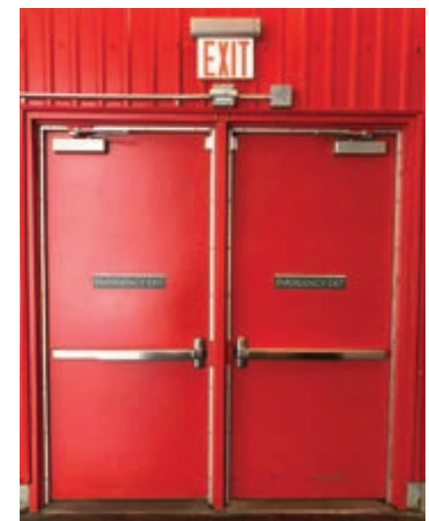
#5077 installed in conjunction with #5077SPB.
