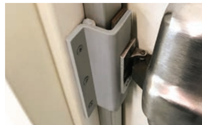
#5077SPB installed at the door strike.
